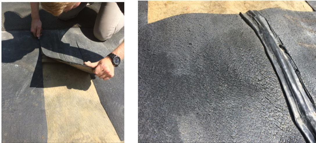
Figure 5, Field sampling of dual track hot wedge fusion seam and fillet extrusion seam
